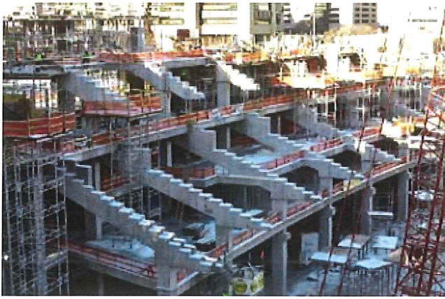
Photo 3: More than 5000 structural precast concrete elements with 28-day minimum strength of 10,000 psi were required for construction of U.S. Bank Stadium
